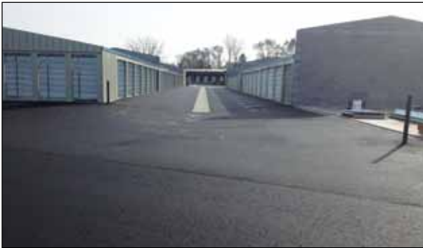
The permeable pavement was designed to capture and retain the water from all runoff events up to the 100-year design storm (4.4 in. of runoff).
